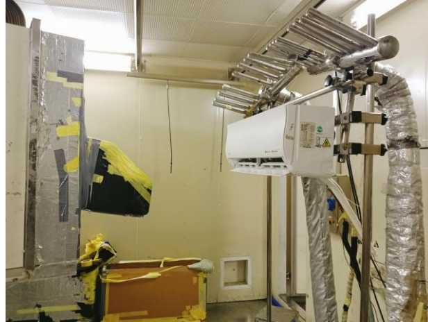
Figure 1. Psychrometric laboratory installation and indoor unit installation
